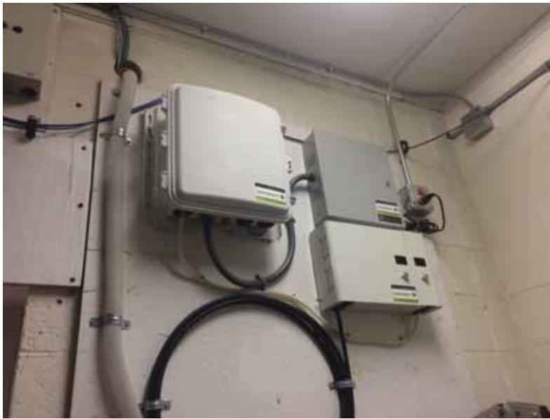
Communications/ Fiber optics
