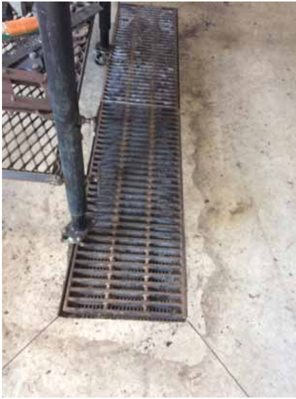
Floor trench drain
