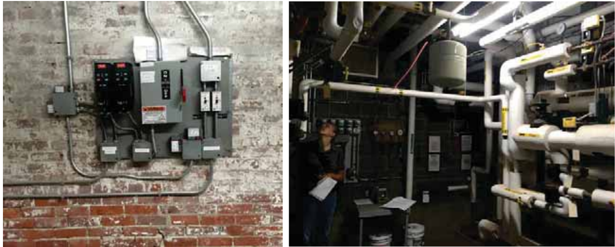
Figure 6 & 7: Basement Electrical and mechanical
