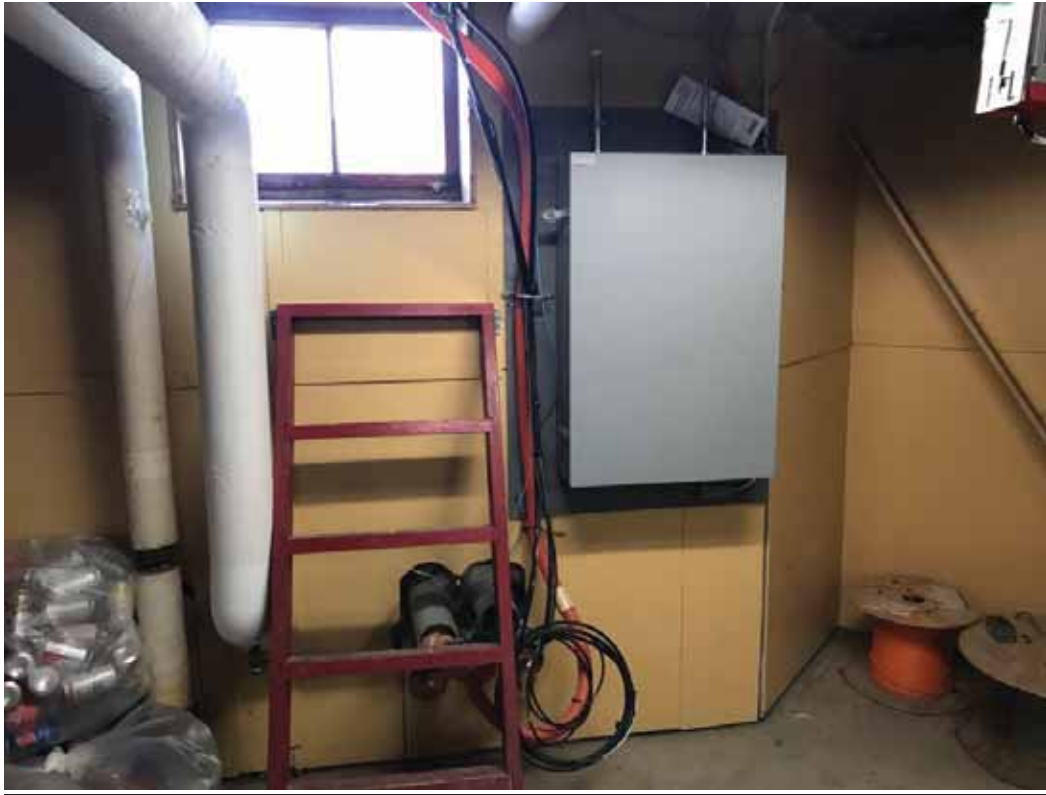
Figure 26: Basement fiber-optic and electrical panel
