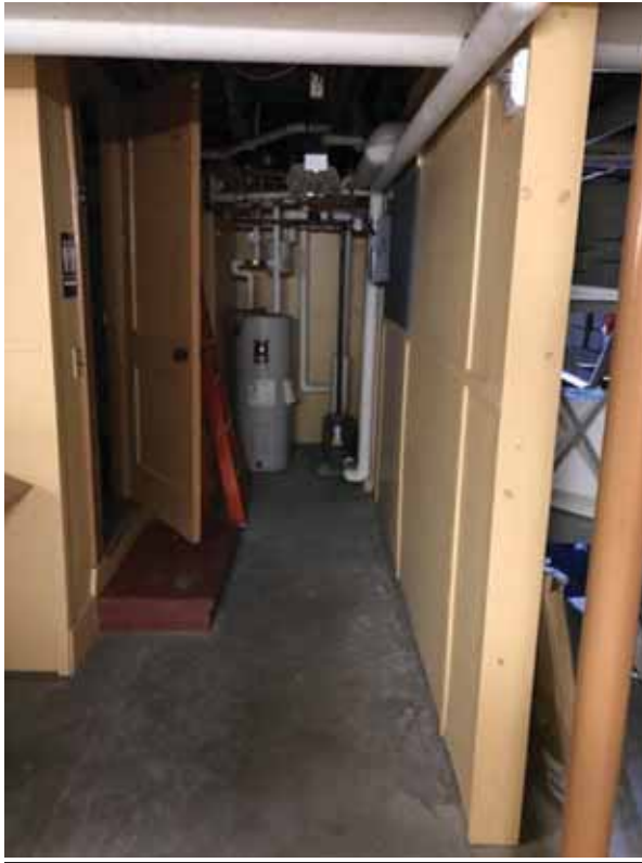
Figure 20: Basement mechanical / hot water heater
