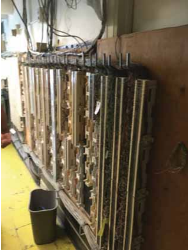
Figure 16: Basement Tel-com equipment
