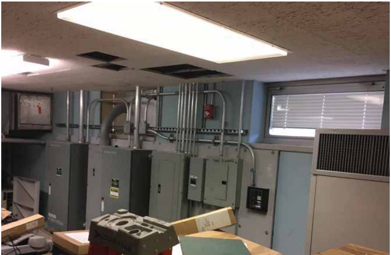
Figure 12: Basement electrical and mechanical equipment.
