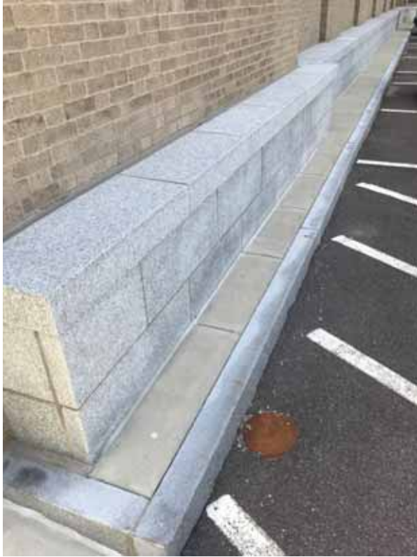
Figure 9: West exterior wall granite base course (appears to be of newer construction)
