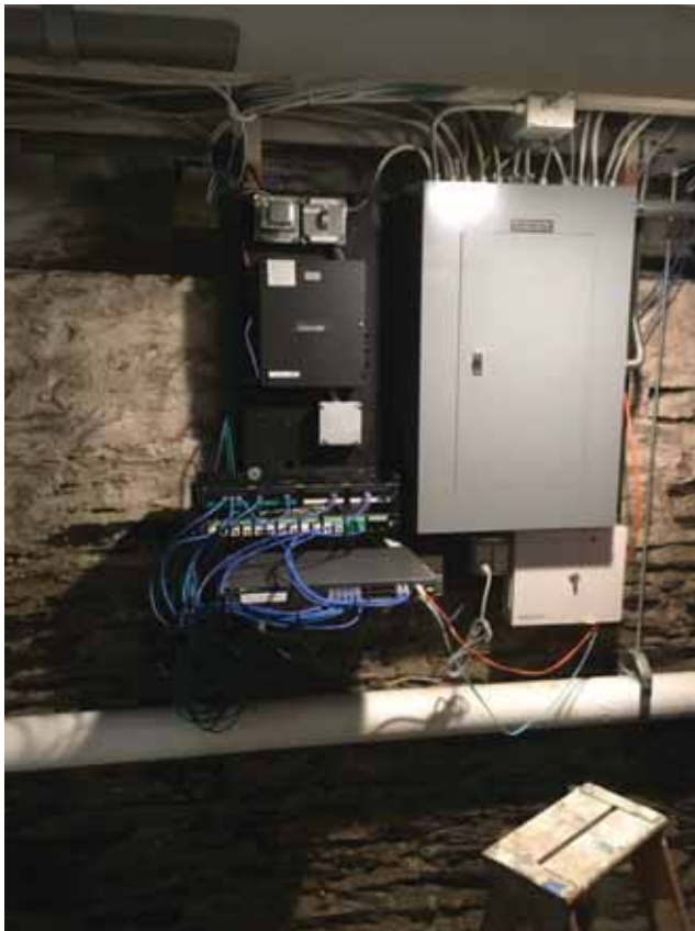
Figure 13: IT, Electrical, Security
