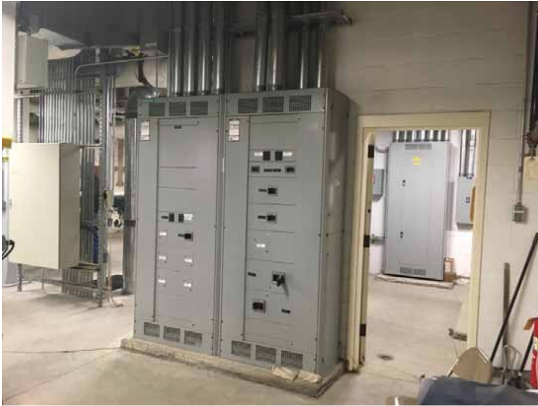
Figure 17: Sub-basement electrical panels
