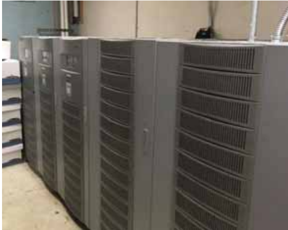
Figure 10: Liebert network power units
