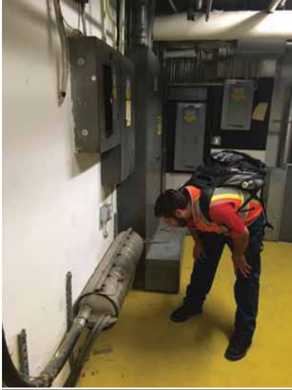
Figure 14: Basement electrical equipment
