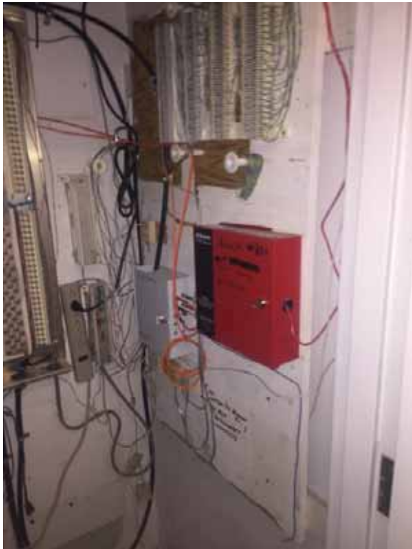
Figure 7: Telcom / Security Panels (Source: MSK)
