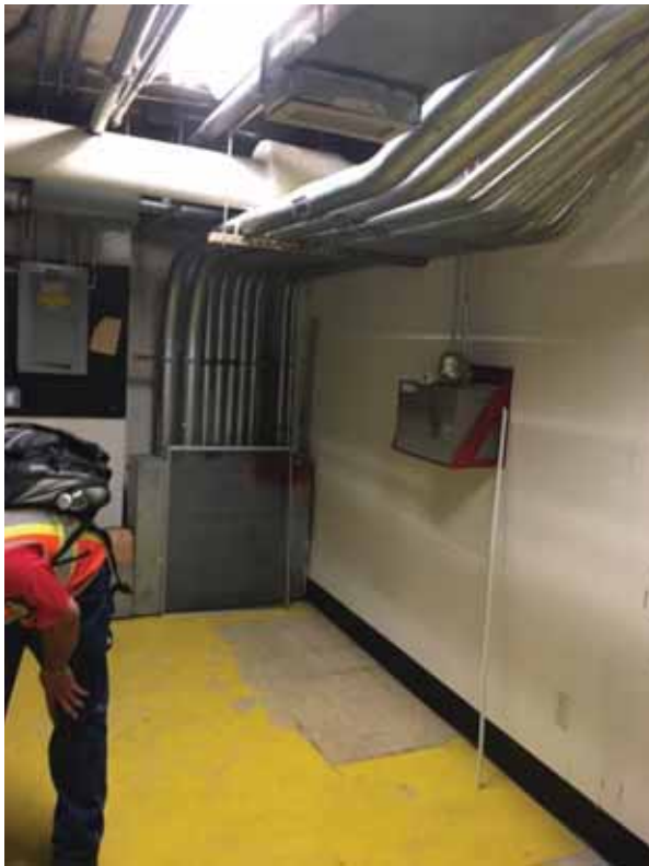
Figure 15: Basement electrical equipment
