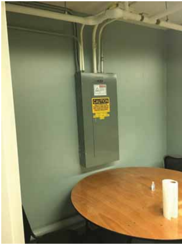
Figure 19: Basement electrical equipment
