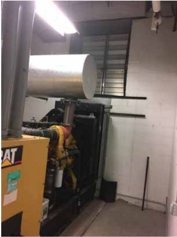
Figure 13: Sub-basement emergency generator
