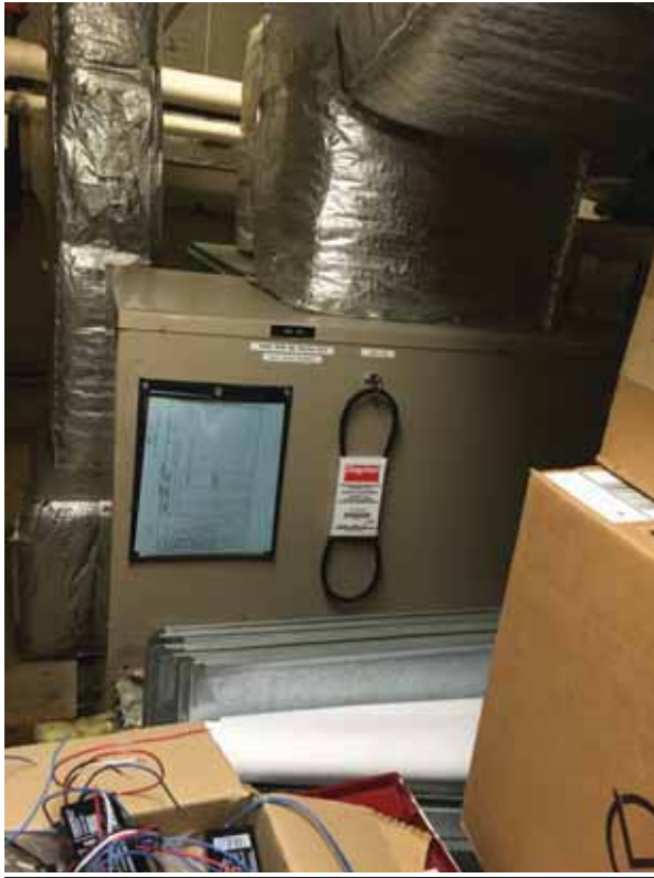
Figure 18: Basement mechanical equipment
