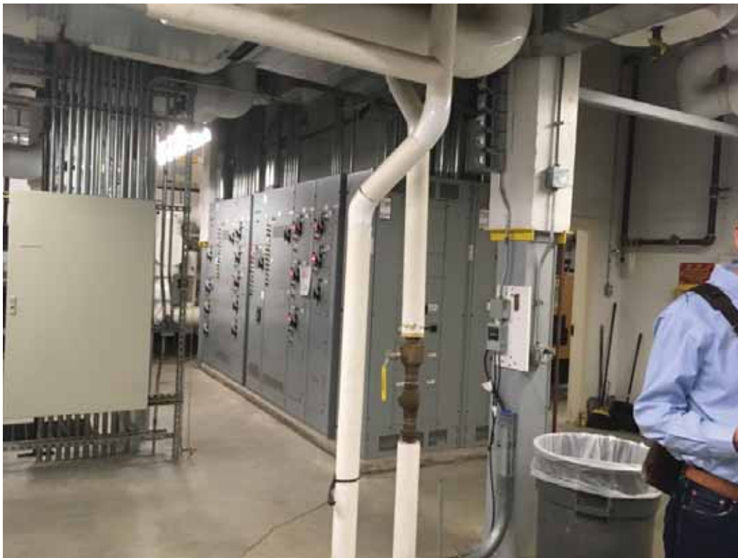
Figure 16: Sub-basement electrical panels
