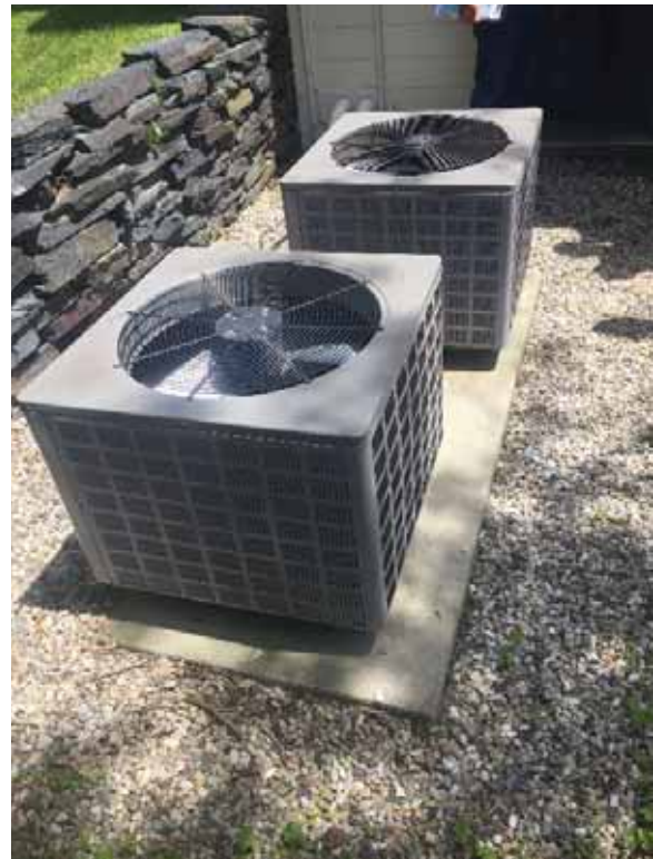
Figure 6: Exterior A/C Units (Source: MSK)
