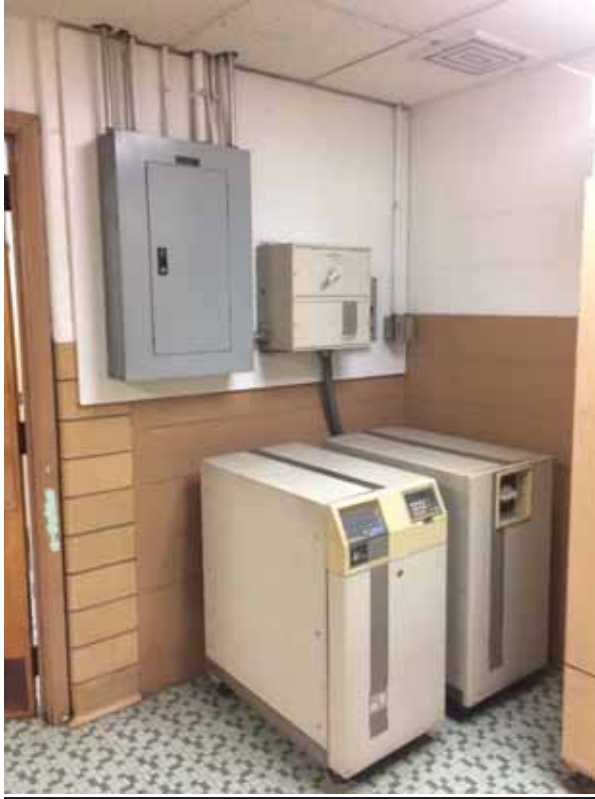
Power panels and fixed equipment
