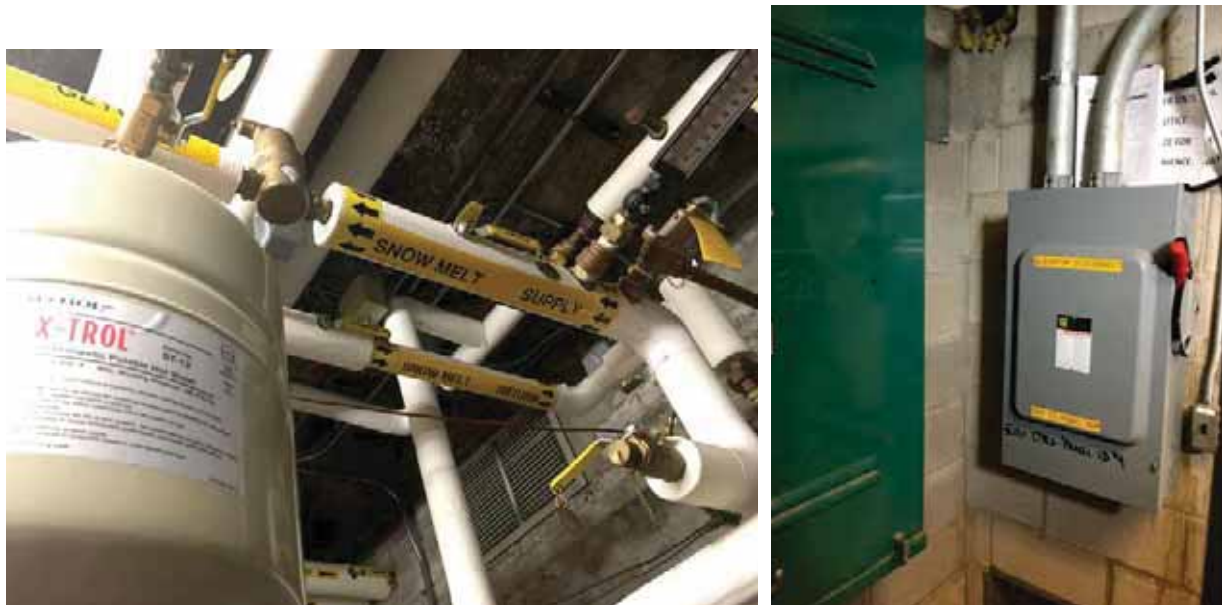
Figure 8 & 9: Basement mechanical and electrical
