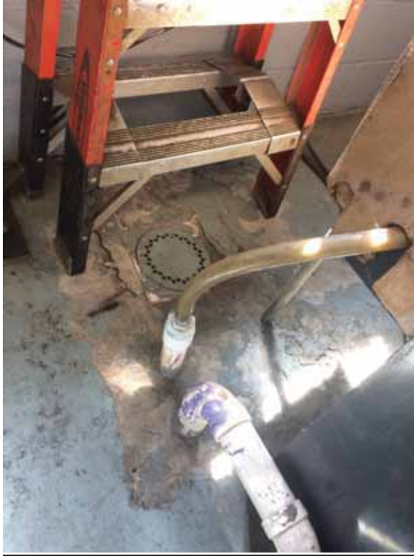
Floor drain and piping
