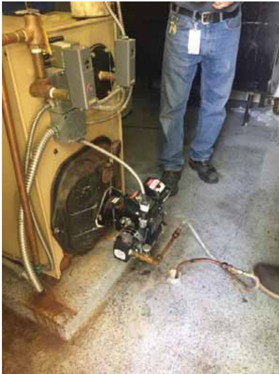
Figure 5: Boiler in Mechanical Room (Source: MSK)
