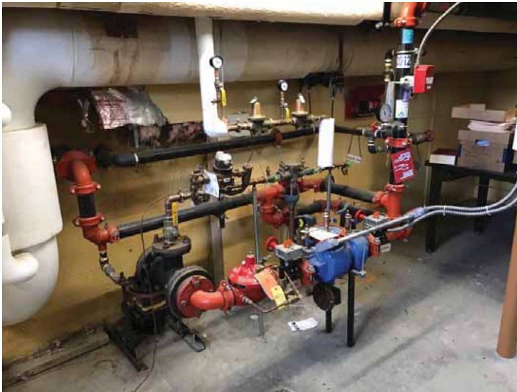
Figure 25: Basement sprinkler riser
