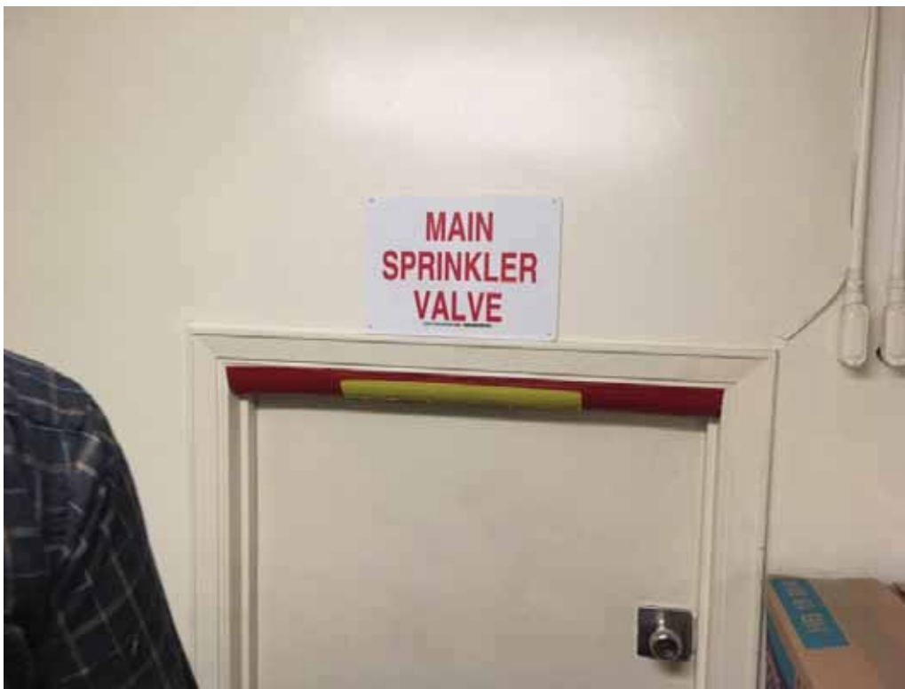
Figure 17: Basement sprinkler room
