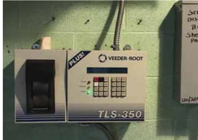
Figure 11: Emergency Generator Tank Monitor
