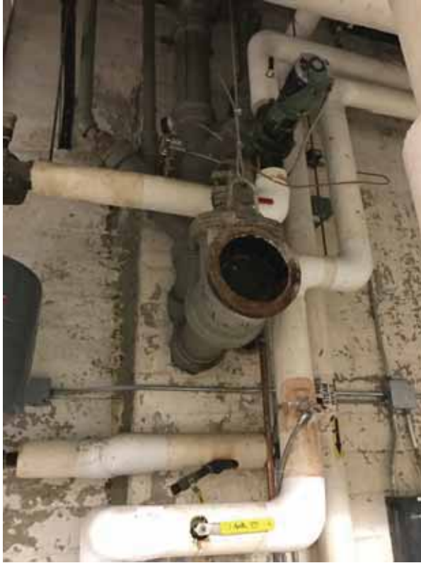
Figure 21: Multiple wall penetrations in sub-basement walls (potential for water infiltration)
