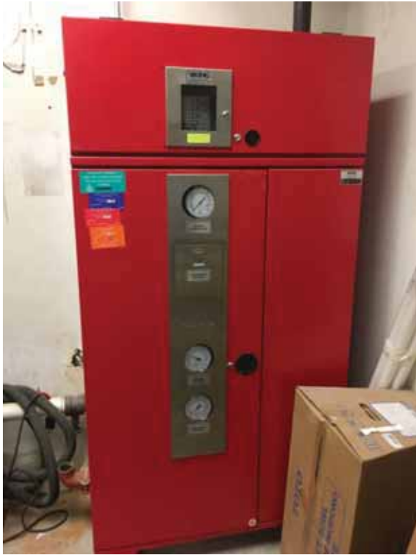
Figure 11: Basement level fire safety equipment
