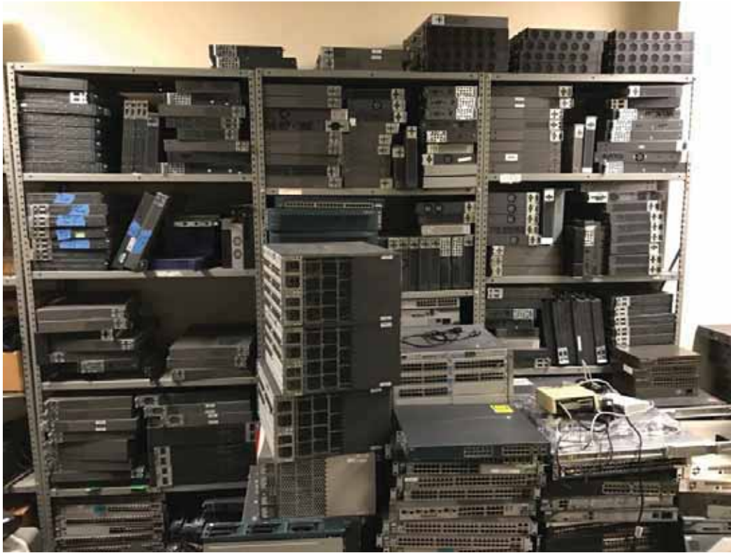
Figure 35: Basement-level storage racks (FF+E is not included in cost opinions)
