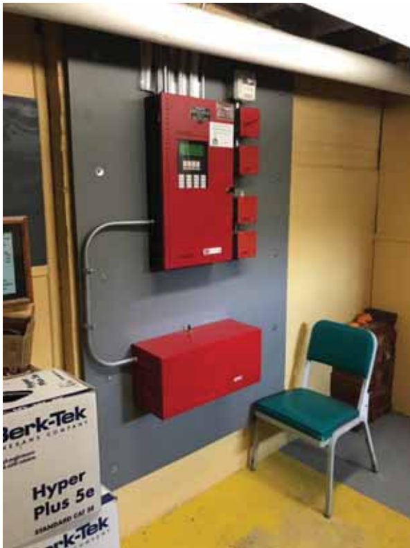
Figure 21: Basement fire alarm panel
