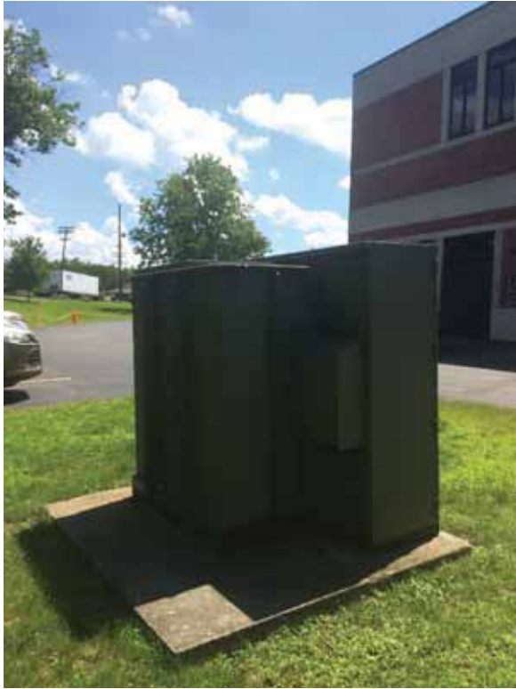
Figure 5: Exterior pad mount transformer.
