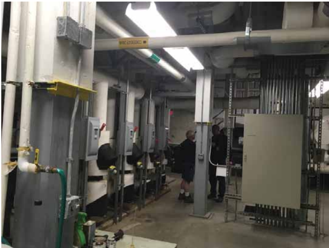
Figure 18: Sub-basement electrical panels / mechanicals
