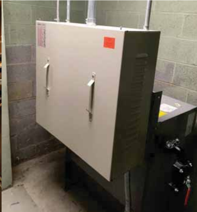
Figure 7: Elevator machine room equip
