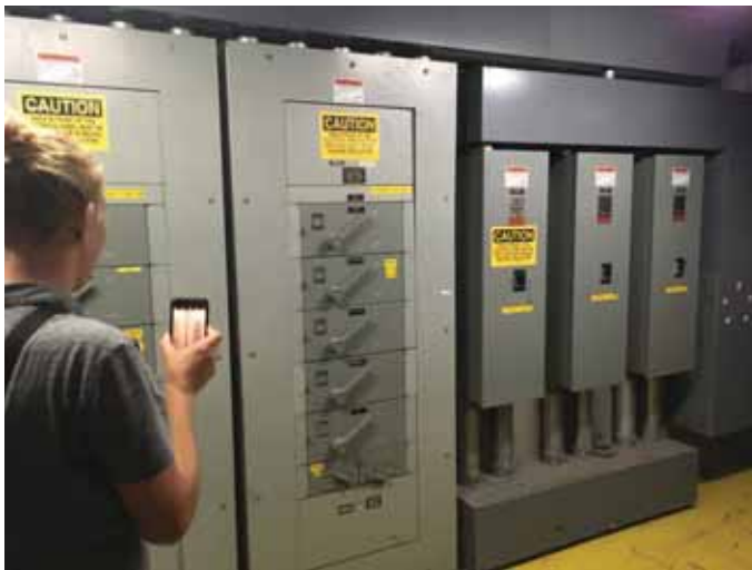
Figure 12: Basement electrical equipment
