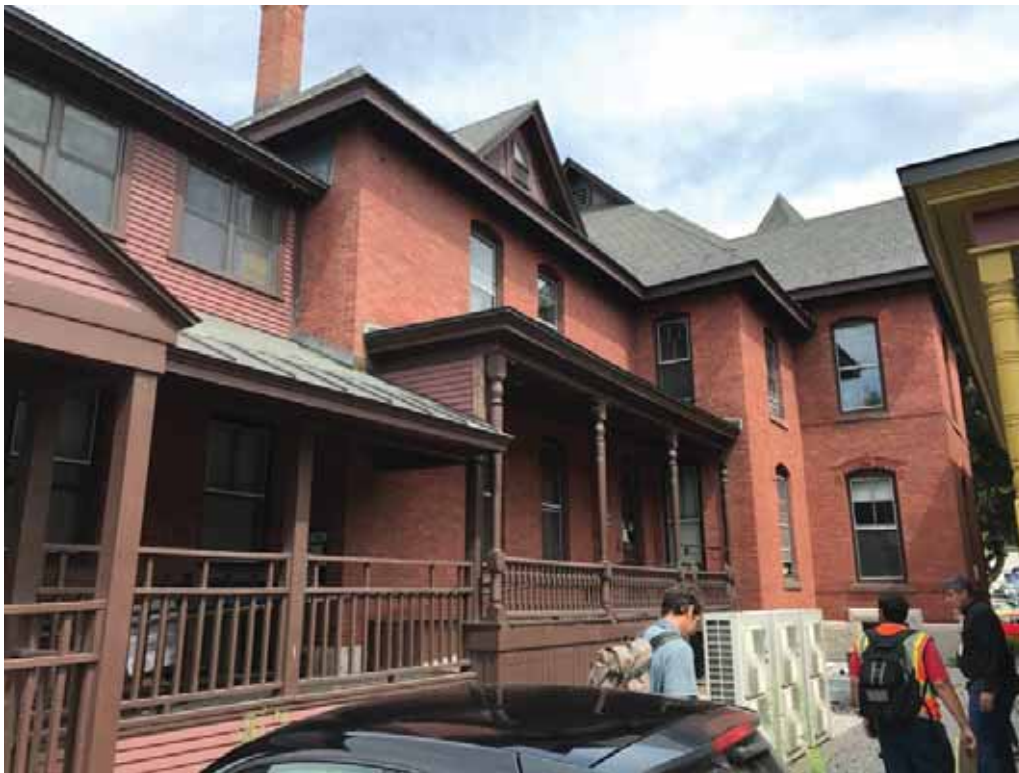
Figure 13: Site mounted split system AC units
