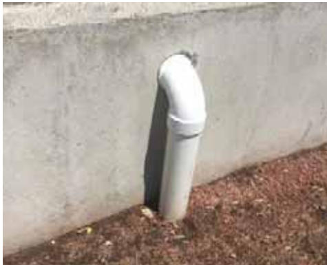
Figure 12: Unsealed exterior wall penetration(s).
