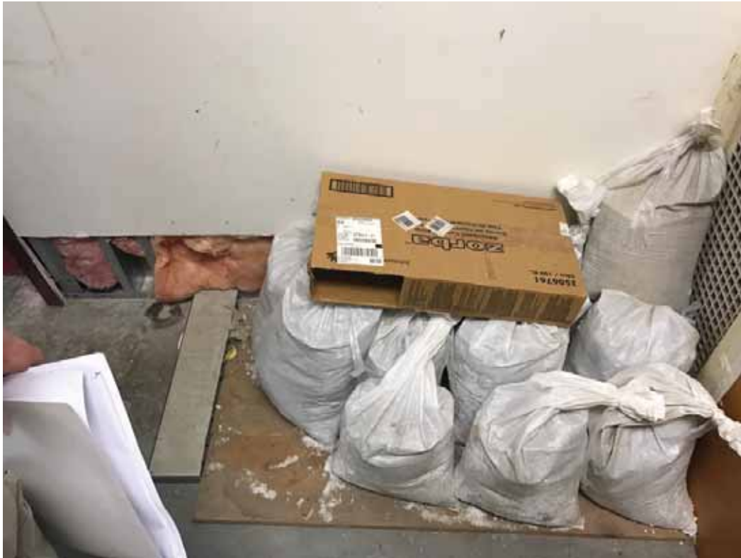
Figure 37: Pre-existing basement-level water damage observed in areas
