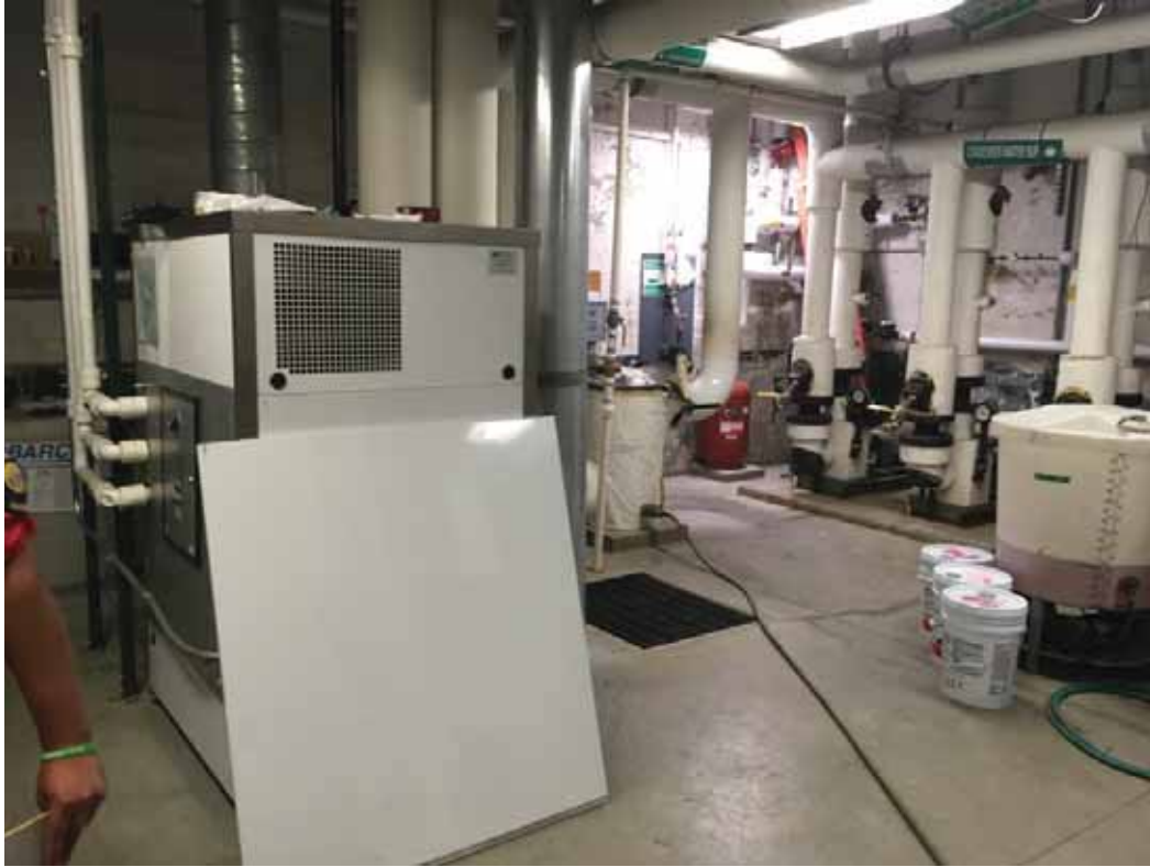
Figure 15: Sub-basement mechanicals and steam
