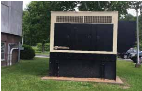
Figure 15: Pad mounted Generator (SE corner)
