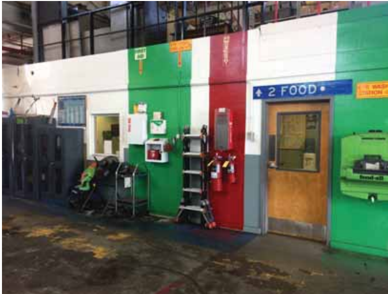
Contents could be hazardous if not addressed prior to flood event
