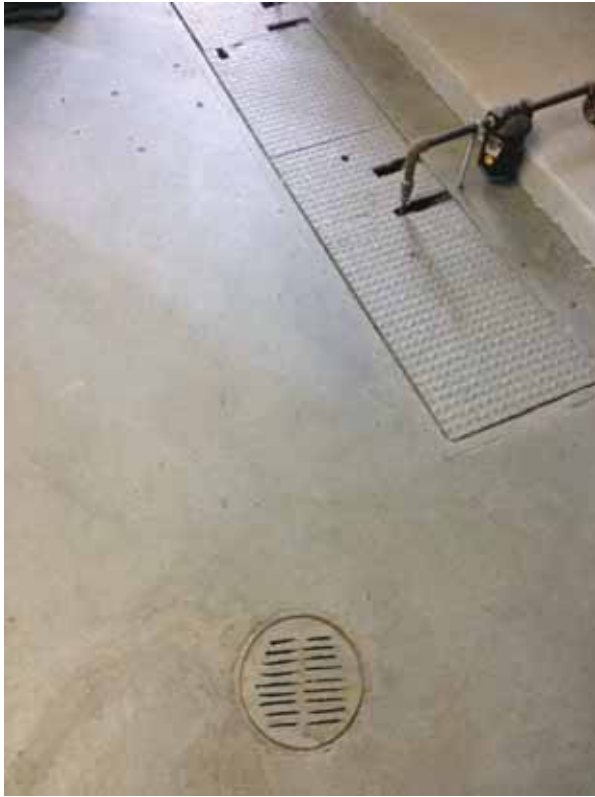
Floor drains and access panel
