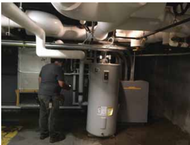
Figure 13: Basement mechanical equipment
