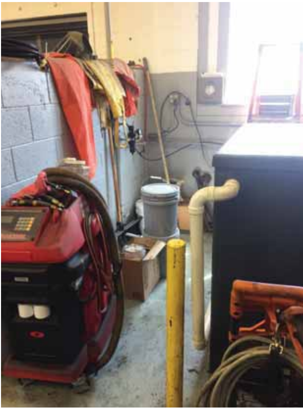
Contents could be hazardous if not addressed prior to flood event
