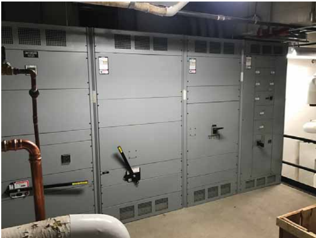
Figure 36: Basement-level water electrical panels
