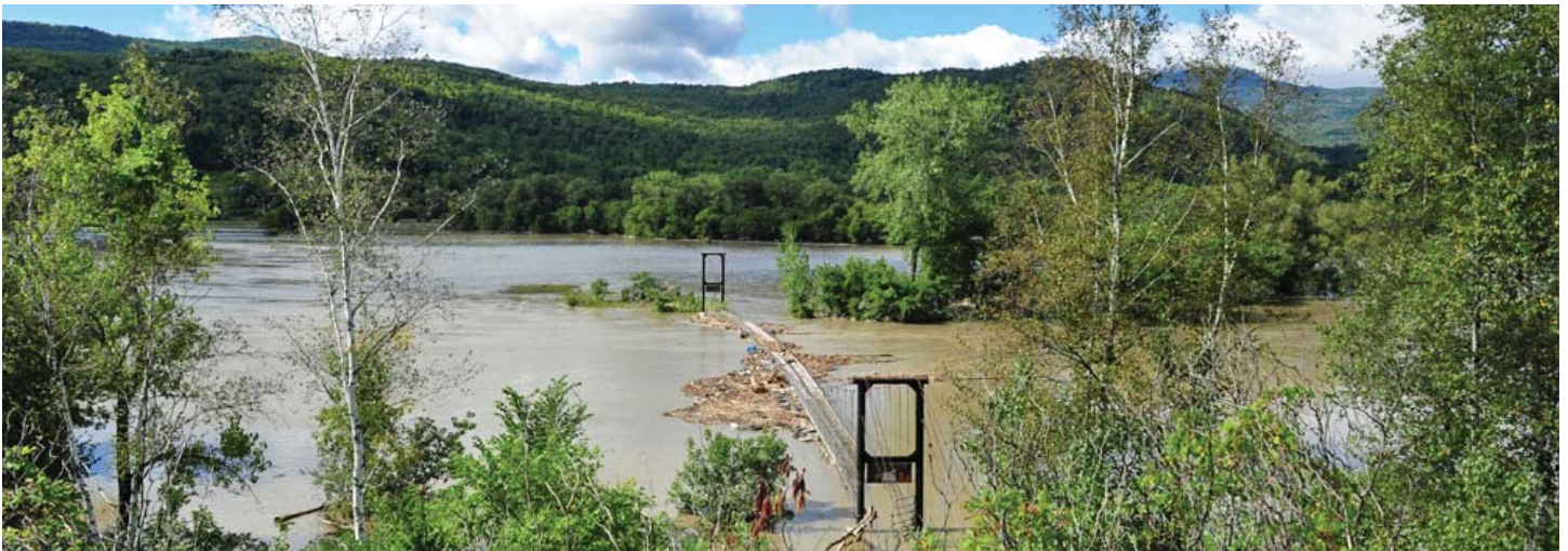
Snowmobile bridge near Waterbury, VT flexes as debris and water rush past following Tropical Storm Irene
