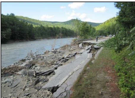
Tropical Storm Irene damage, 2011 Photo credit: Joe Flynn, Department of Public Safety
